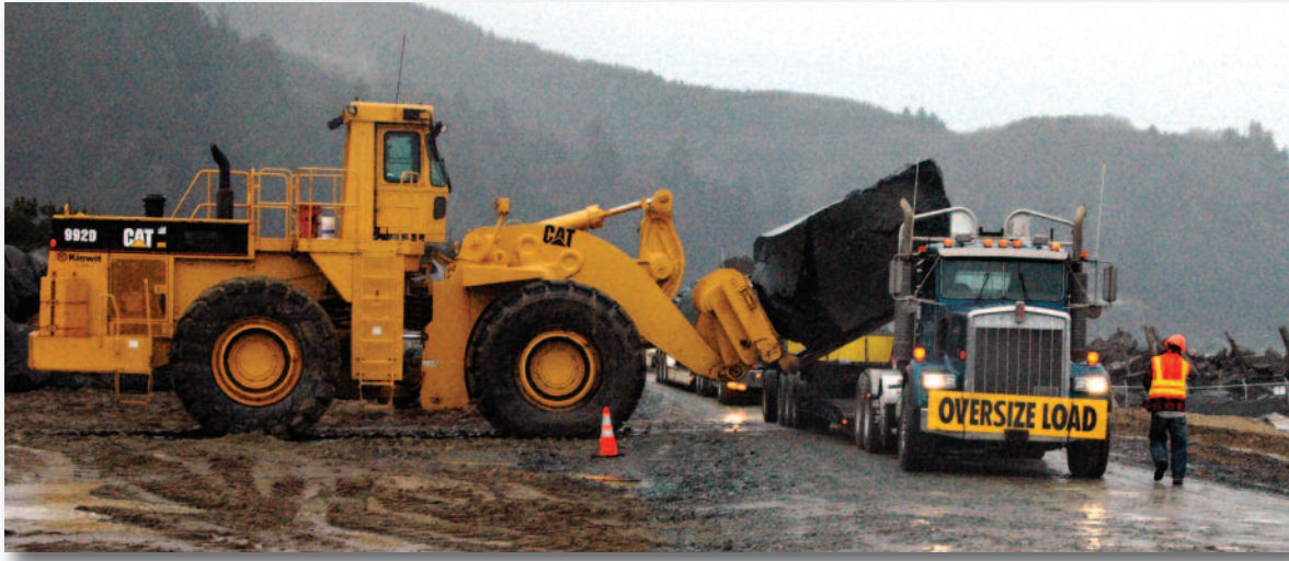
A giant forklift removes a huge boulder from an incoming truck at the Barview Jetty staging area.
